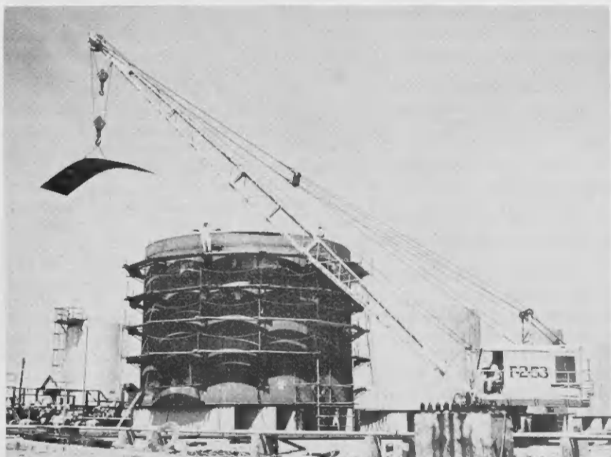
ON THE business end of a Lago crane is a sheet of steel for a nearly-completed storage tank being erected in the vicinity of tank No. 495. DEN GARA di un grua di Lago ta un plachi di staal pa un tanki casi cla cu ta worde lamtá den proximidad di tanki No. 495.
